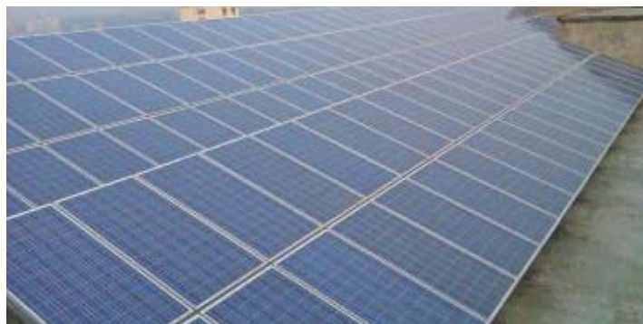
A portion of BBS Solar panels are seen at rooftop of Parishankhyan Bhaban
